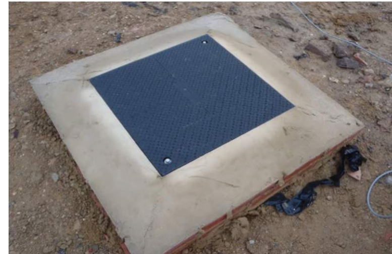
Injection Lines grouped in Chamber for future access
