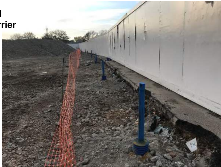
Permeable Reactive Barrier / Treatment Zone
