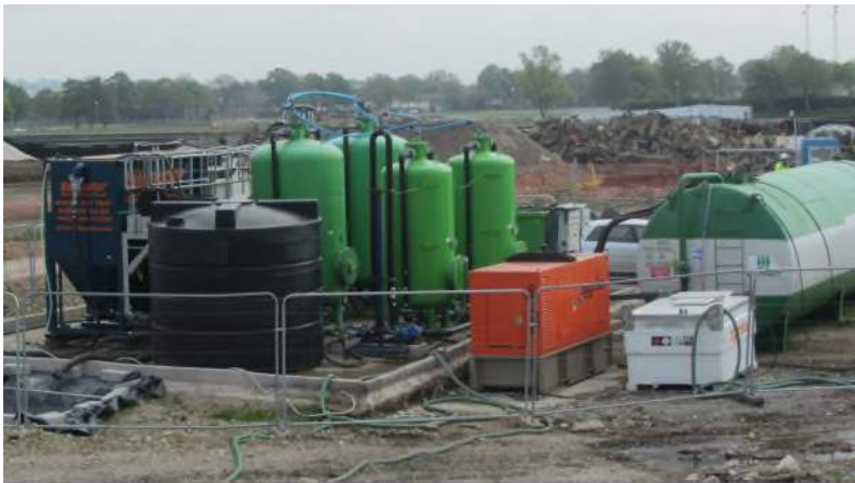
Groundwater Treatment System
