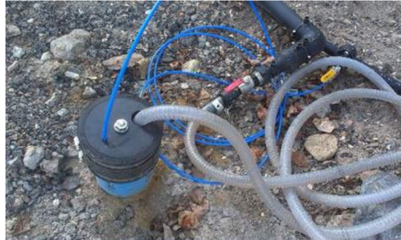
Groundwater Pumping & Recirculation
