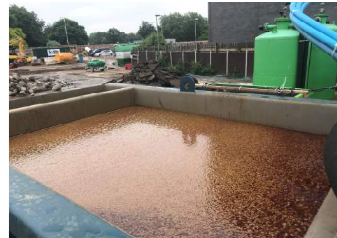
Groundwater Treatment Plant
